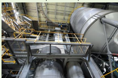
Figure 1 Circulation fluidized bed combustion furnace facility
