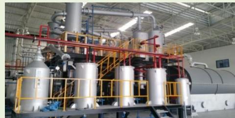
Picture 3 Waste plastics power generator
